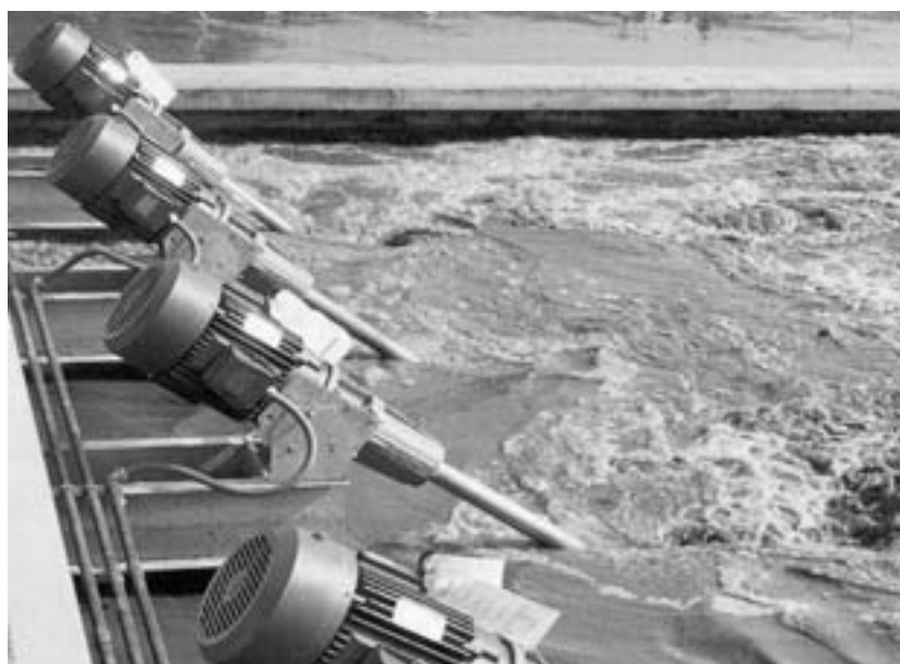
Figure 8-38(l) Alternative device for aeration: Fixed-mounted, aspirating aerators. (Photo courtesy of Eimco Process Equipment, a Baker Hughes Company.)
