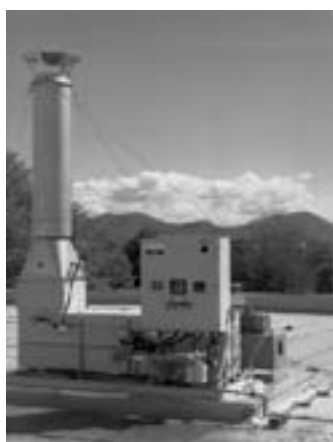
Figure 10-15 Photograph of an operating catalytic oxidizer. (Courtesy of Stealth Industries, Inc.)
