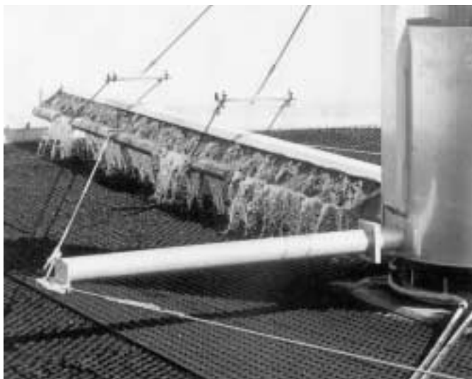
Figure 8-47 Photograph of rotary distributor for trickling filter. (Courtesy of U.S. Filter/General Filter.)
